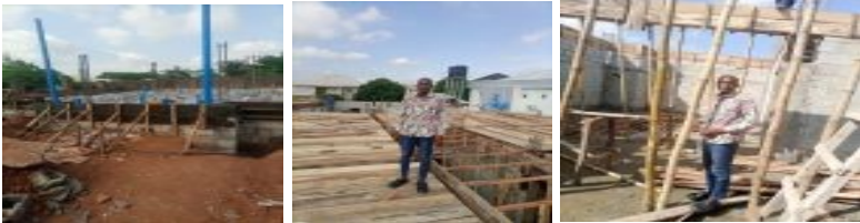
Figure 1 a) formwork for plinth b) decking for upper floor c) formwork for lintel
