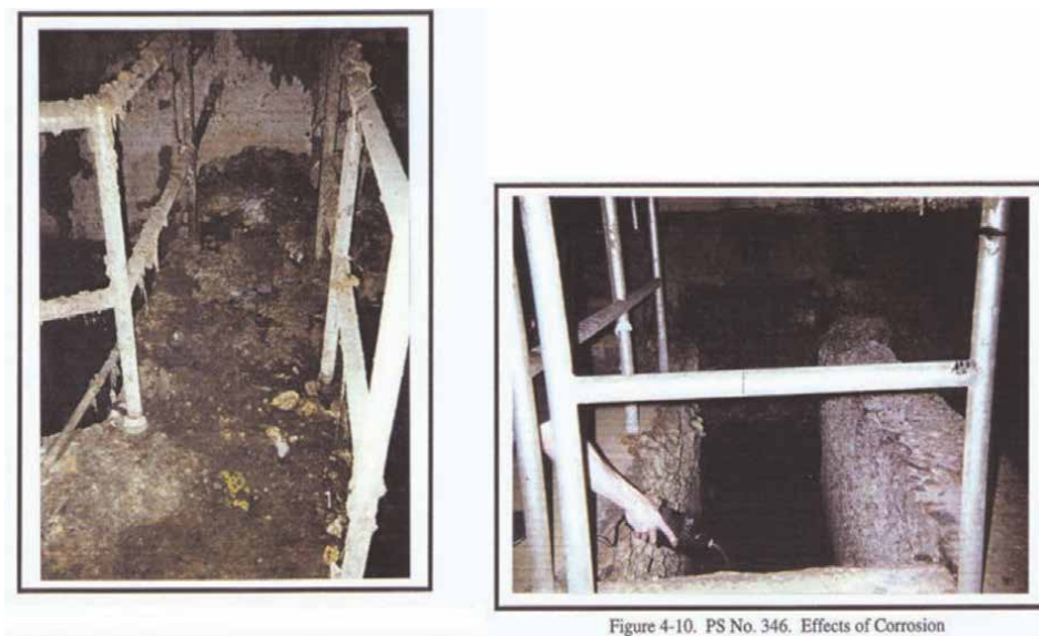
Figure 4-10. PS No. 346. Effects of Corrosion
