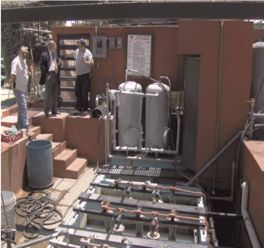
Figure 16. Picture of electroflocculation technology (copyright of Reingeniería en Saneamiento ltd).
