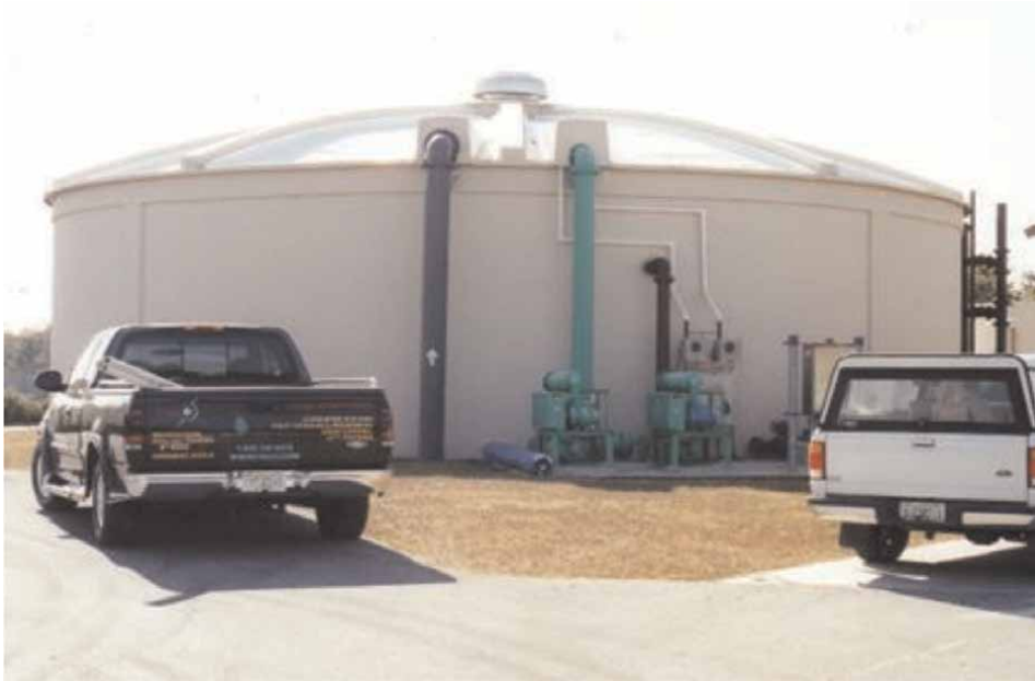
Figure 9. Sludge thickener facility (with TRIO 3 permitted authorization).
