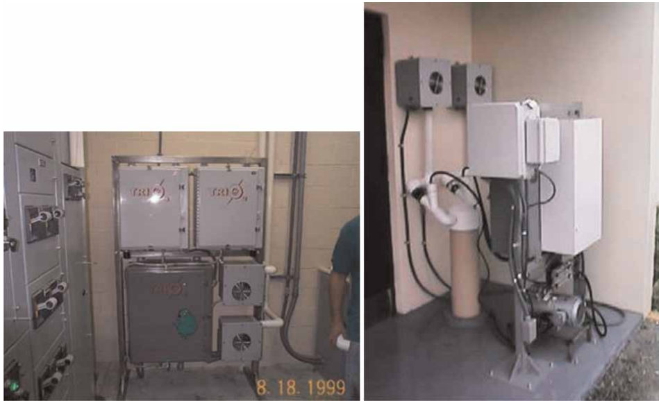
Figure 5. Ozone generator (gas bust 2000 displayed with TRIO 3 permitted authorization).
