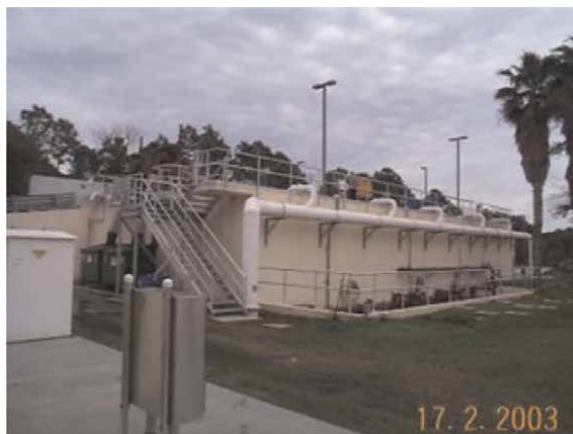
Figure 7. Septage tank with a gas buster unit installed (with TRIO 3 permitted authorization).
