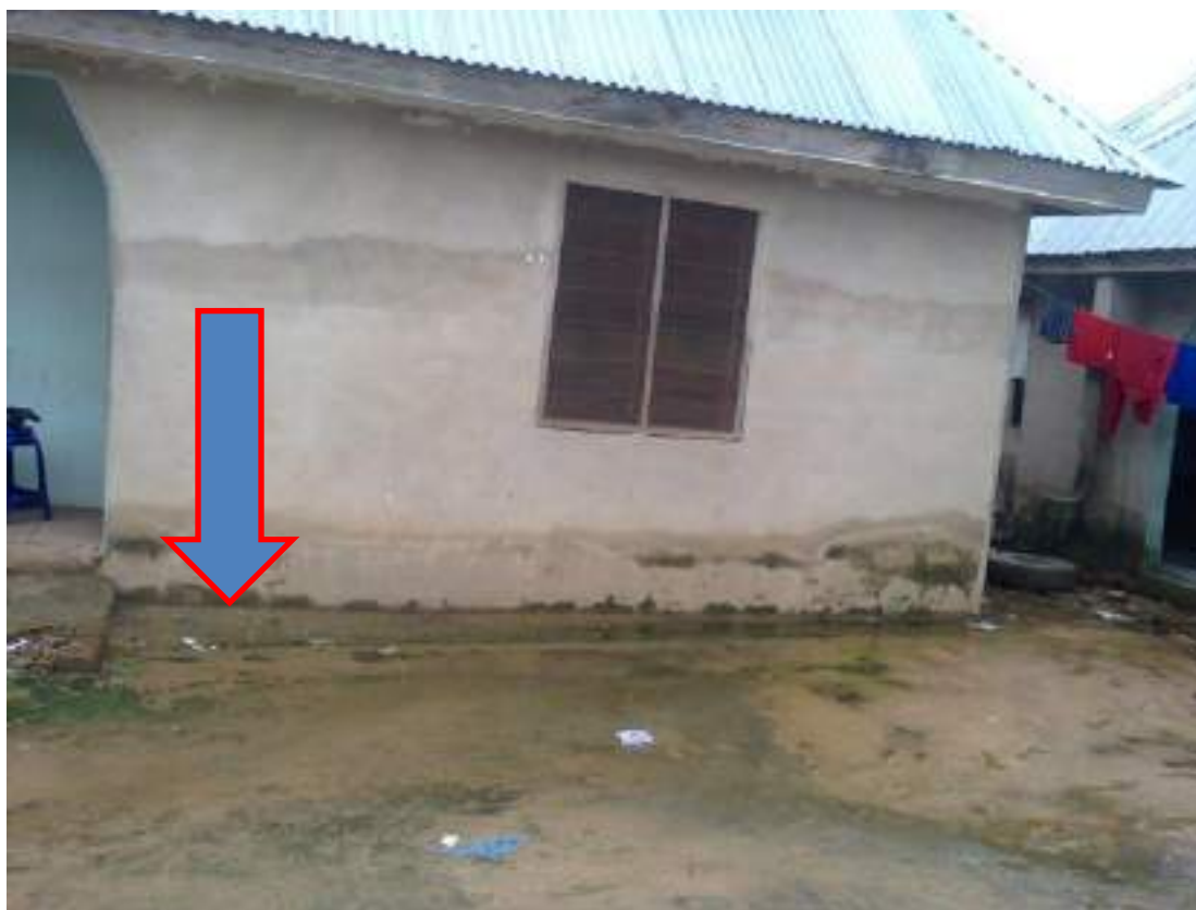
Fig. V: imprint of flood on building’s wall, signifying the level or height of flood waters at the time of impact. (Source fieldwork)
