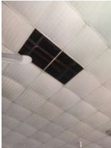
Picture 4: Damaged ceiling
