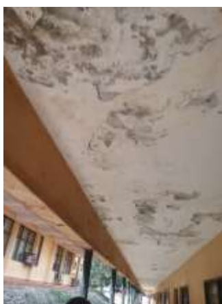
Picture 2: Faded paint and holes
