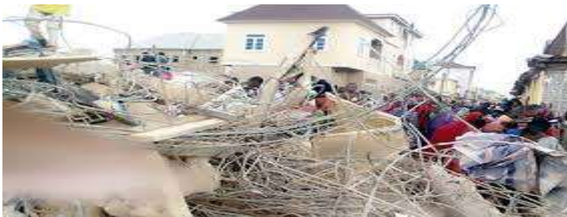
Plate 2 shows Three-storey building collapse in Dilimi Community of Jos North Local Government Area of Plateau. Confirmed by NEMA (2019).
