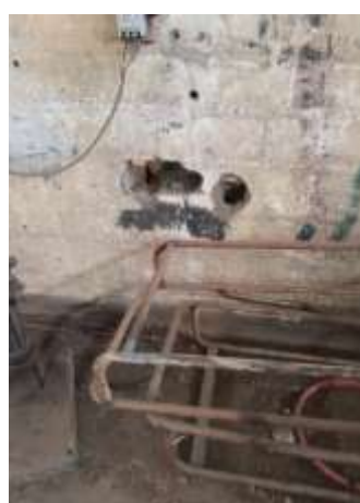
Picture 3: Faded paint and holes on wall
