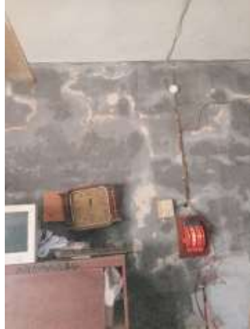
Picture 5: Exposed wire and faded paint
